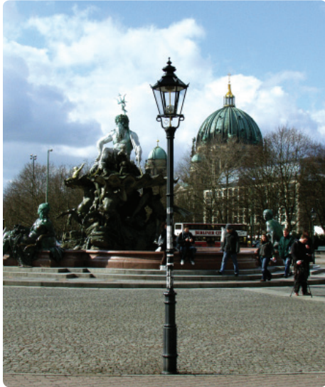
Braun's LED-driven street lamps installed on Berlin's Alexanderplatz public square
